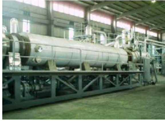
Equipment in Operation
